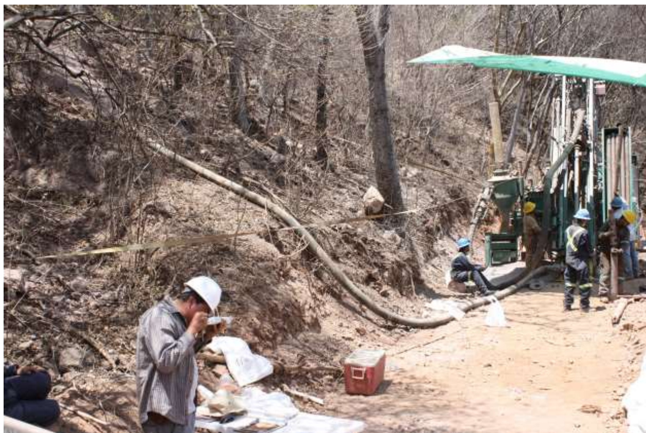
Figure 1. RC drilling utilising a skidder type RC rig which commenced drilling ranked targets from Sunday 29 th May.
